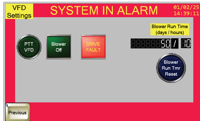
FIGURE 14b. VFD Screen in Alarm
